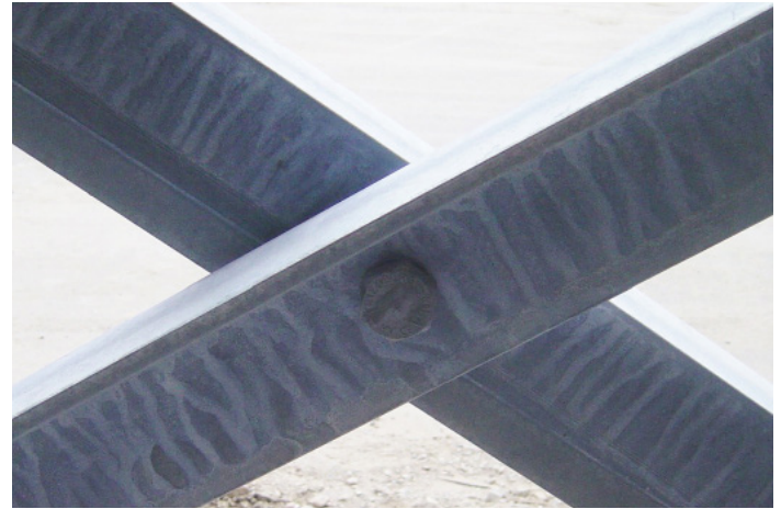
Fig 1. Wet storage stain formed on galvanized surface
