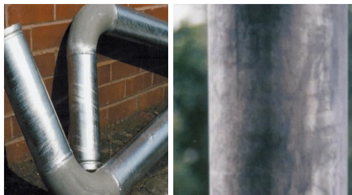
Fig 3. Examples demonstrating how the silicon content of steel can cause changes in the appearance of a galvanized coating.
