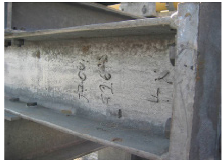
Fig 2. Uncoated areas due to paint markings not removed prior to galvanizing
