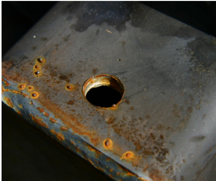
Fig 1. Weld spatter present on steel before galvanizing
